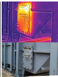
Thermal image of exhaust access door.
