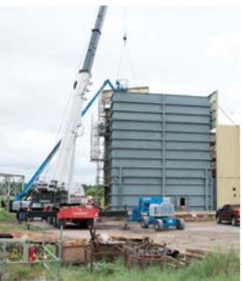
501D exhaust stack and silencer.
