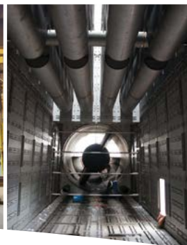
Internal view of Schock Liner System.
